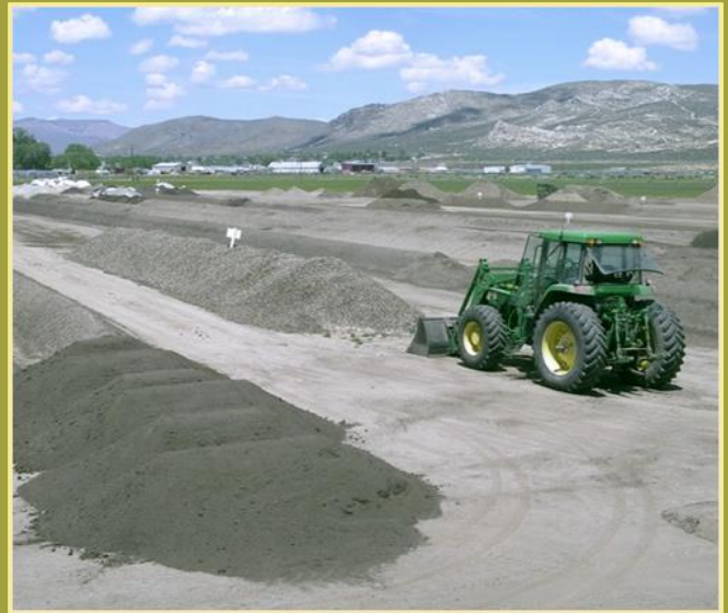
Managing compost at the Northern Nevada Correctional Center. Photo from Craig Witt.
