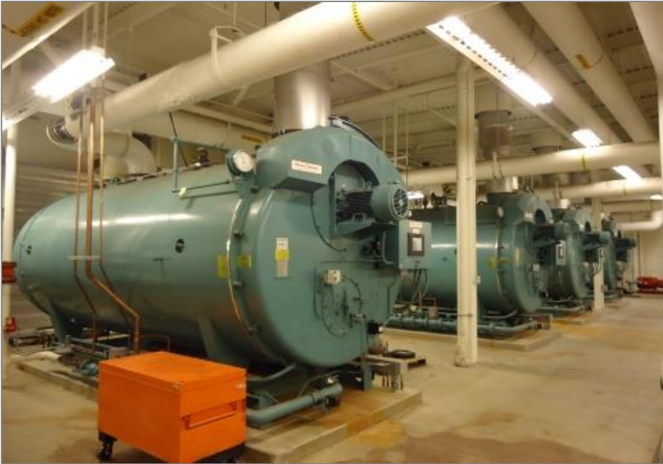
The Peppermill's four boilers once consumed $2.2 million dollars per year in natural gas. Heating the Peppermill with geothermal energy reduces the Peppermill's CO 2 emissions by 12,000 metric tons per year. Photo from the Peppermill.
