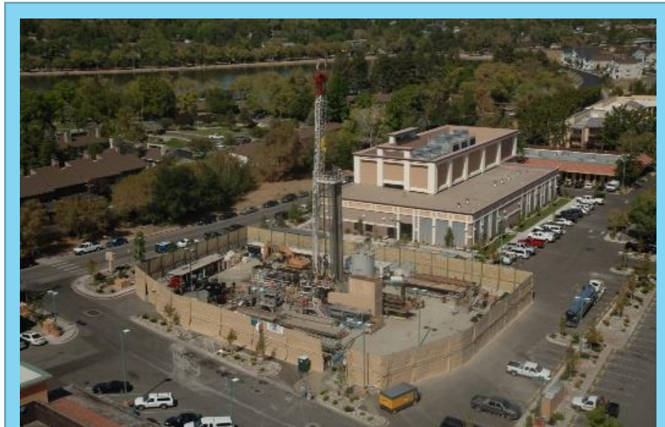
The Peppermill's production well #8 took 28 days to drill and reaches 4,421 feet deep, into 174°F water. Photo from the Peppermill.
